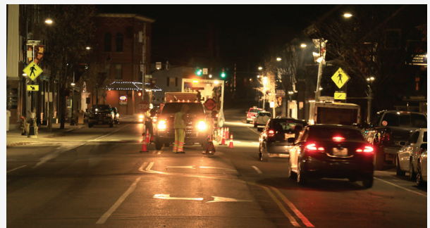
Small construction footprint needed by UV-CIPP process allows streets to remain open.
