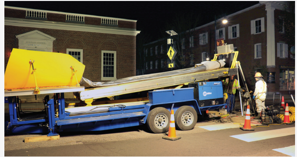
UV-CIPP liner preparing to be inserted into the egg-shaped brick sewer, through a manhole. No digging was required.
