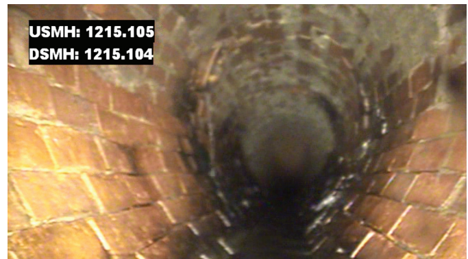
Before: CCTV inspection of the egg-shaped brick sewer prior UV CIPP lining process.
