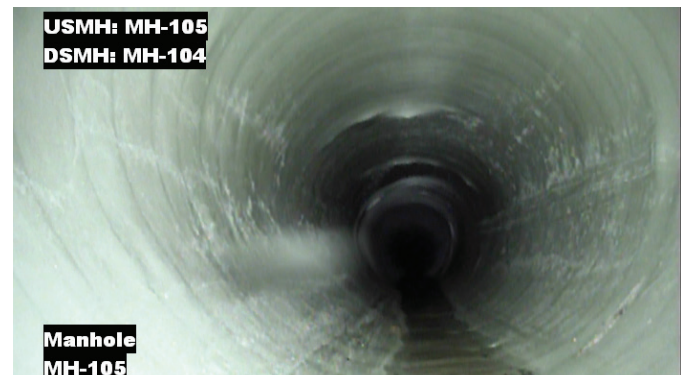
After: Post installation footage shows a complete cure and how the UV cured liner conforms to shape of the brick sewer.
