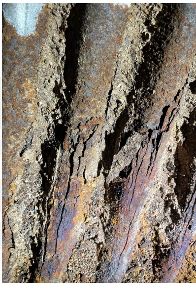
Closeup of the decayed CMP
