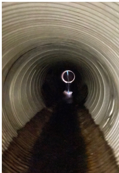
Pipe deterioration on the invert
