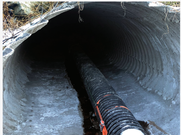
A completely internal bypass system, including a bulkhead, was installed to capture and control stormwater flow during the project.
