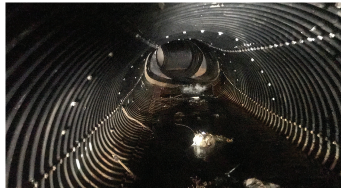
Collapsing culvert prior to QLS installation.
