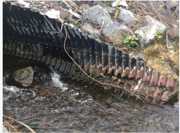
Corrosion in the invert weakened the culvert and also caused severe I/I.
